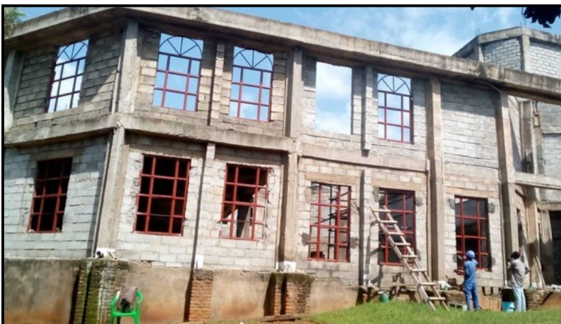
The windows are installed at Sadzi. We thank you all, at Faith, for your hand.
